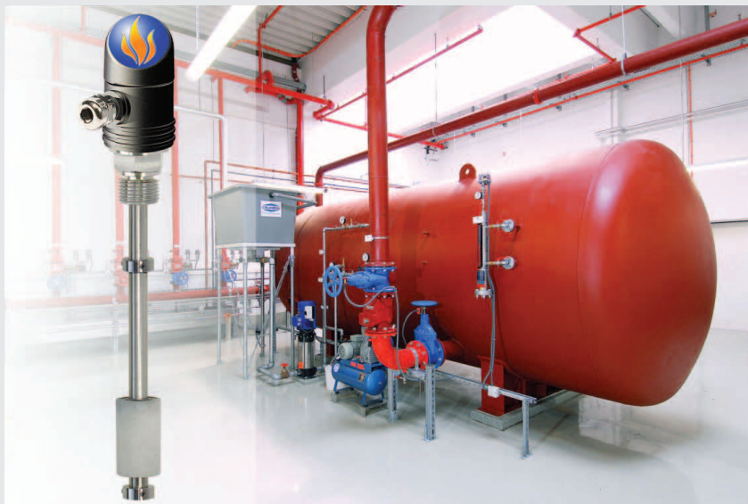
Water tank level monitoring with customized MELS-F level sensor.
